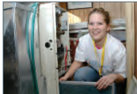
Volunteers helped improve the energy efficiency of 100 homes in Moose Jaw, through the first-ever Share the Warmth Home Energy Efficiency Project.
