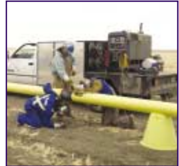
Saskatchewan contractors have benefited from TransGas' Shackleton investment. In 2003, Carson Welding and Maintenance (pictured here), a Saskatchewan-based company, installed 52 kilometres of four, six and eight-inch pipe in the Shackleton area.
