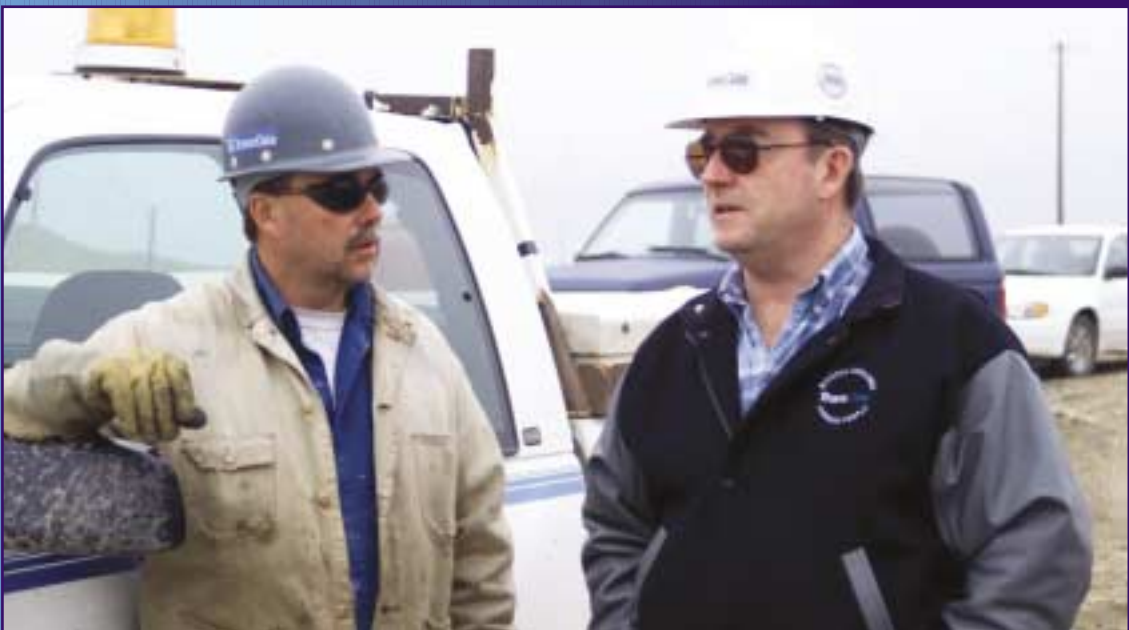
Danny DeBolt, Gas Construction Foreman (left), and Dave Pahl, Superintendent of Pipeline and Storage Engineering (right), oversee pipeline construction in the Shackleton Reserve Area, October 2003.
