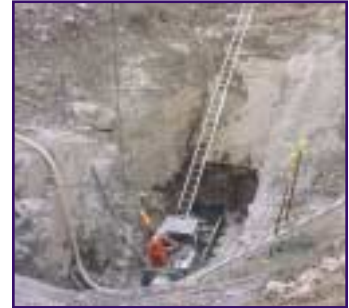
In 2003, Heritage Gas connected the existing natural gas distribution infrastructures in Burnside Industrial Park and Crichton Park by boring underneath Highway 111 in Dartmouth.
