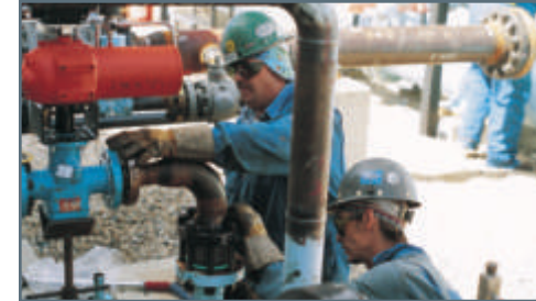
Throughout 2005, the Corporation made a variety of capital investments to maintain its extensive natural gas infrastructure. One of these projects involved replacing aging above-ground piping and valves at the Piapot compressor station.
