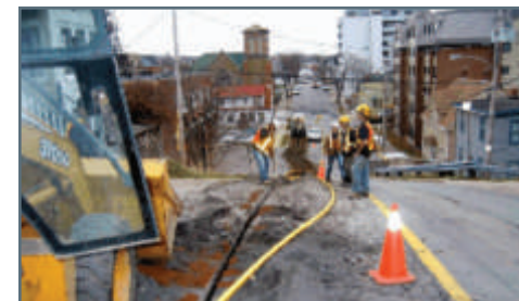
In 2005, Heritage Gas used a variety of construction methods to expand its natural gas distribution infrastructure. Pictured here, a crew uses a rock wheel trencher to install a section of two-inch polyethylene pipe to serve new customers in Dartmouth. More commonly used construction equipment included backhoes, rock breakers and track-mounted excavators.
