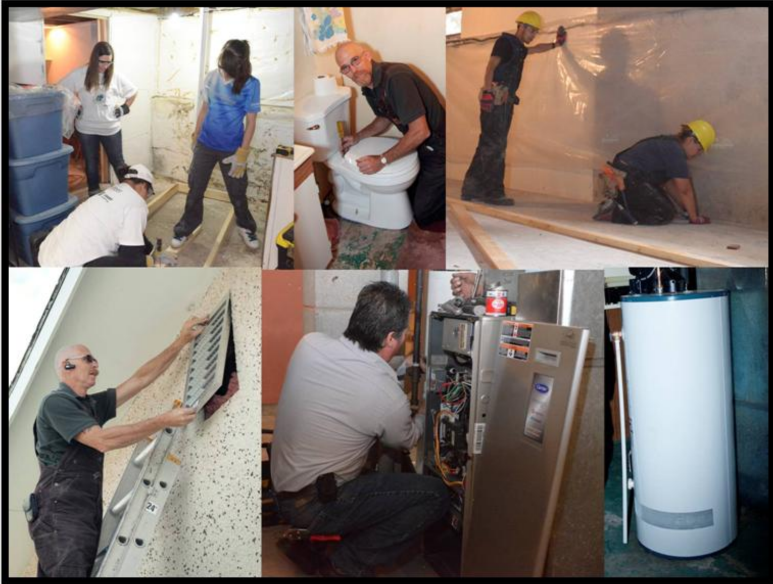
Brand new ENERGY STAR® furnaces, new water heating systems, low-flow toilets and new ventilation units were some of the many products installed in the homes during the energy efficiency makeovers.
